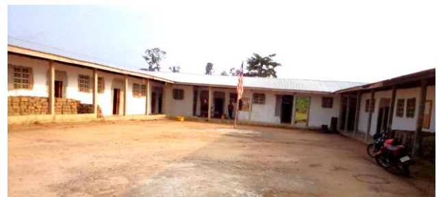
Cement blocks are ready for building a computer lab at Flanagan UMS in Fish Town, River Gee County, March 13, 2023.
