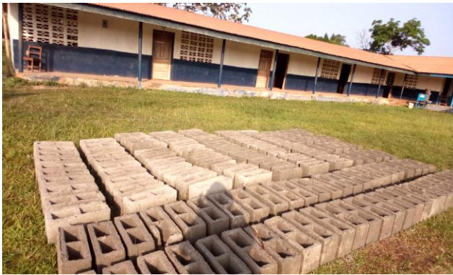
Cement blocks for the fence were molded on the campus of Zwedru UMS, March 9, 2023.
