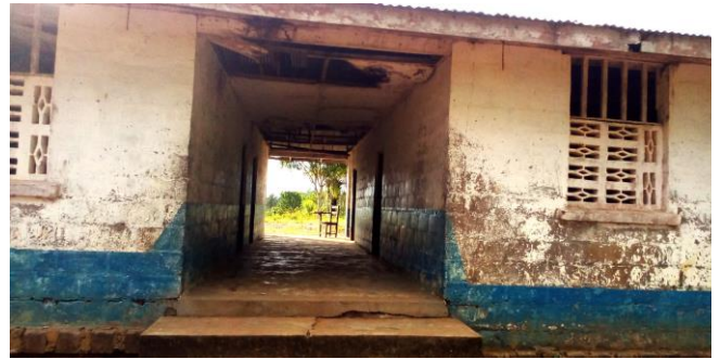
Mary Allen UMS in King William's Town, Sinoe County, March 27, 2023. Renovation of the building has started.
